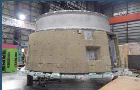
Gas Turbine Exhaust Manifold Insulation
